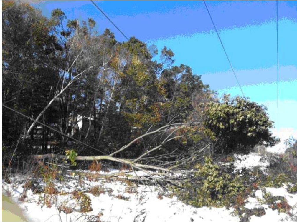
Figure 13: Trees Fallen on 115kV Line in Connecticut
